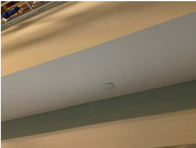
Typical fire sprinkler finishing
