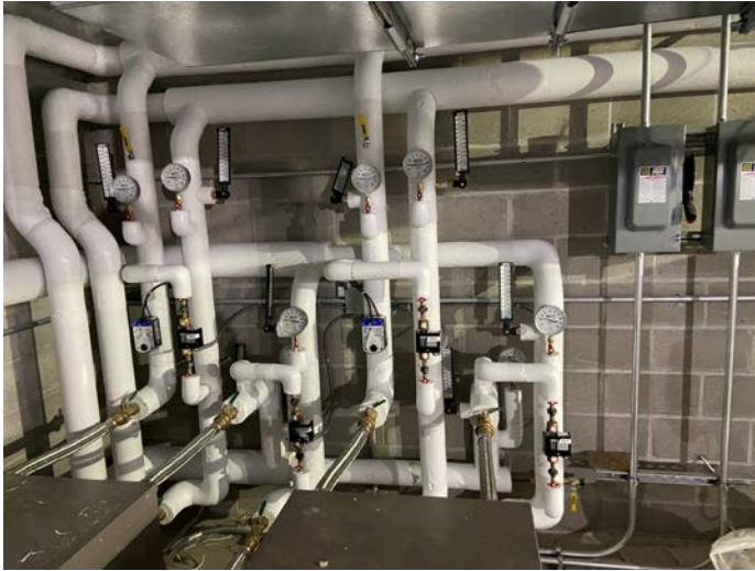
Mechanical mezzanine pipe insulation
