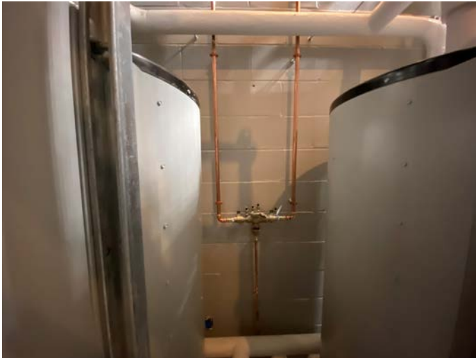
Backflow preventer behind water tanks moved down and bypass removed. Water dept coordinated
