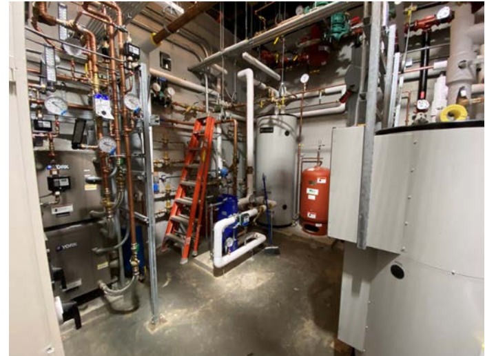
Overview of mechanical room
