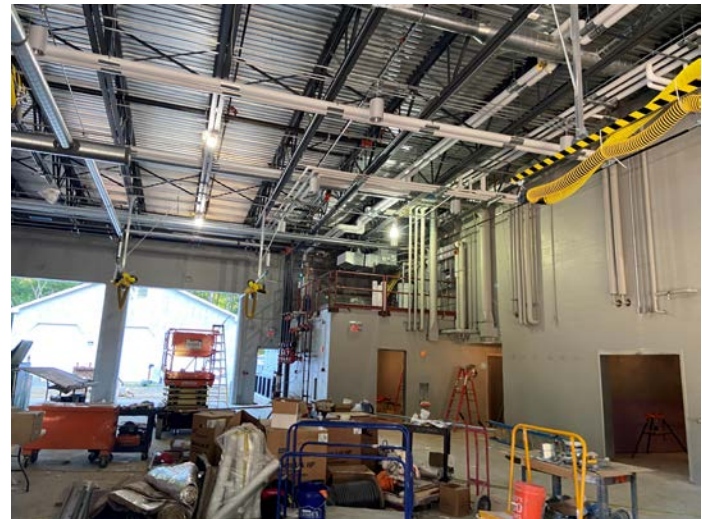
Overview of apparatus bay
