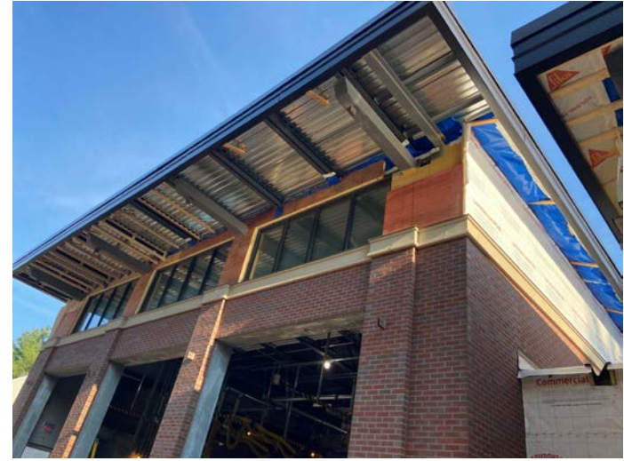
Hunter panel and soffit blocking installation at south side of apparatus bay
