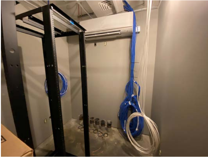
Telecommunication wires at IT/server room
