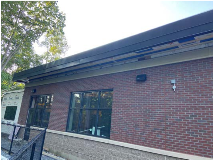
Exterior electrical fixtures on northeast side of building
