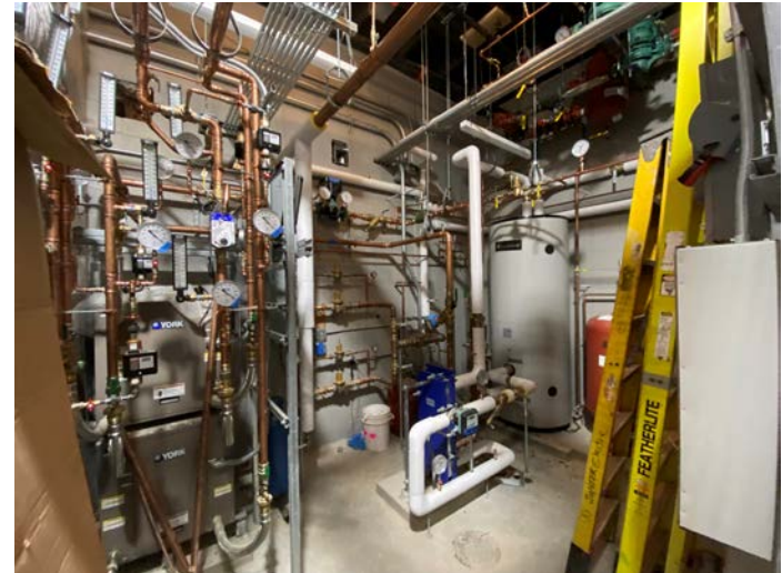
Overview of mechanical room
