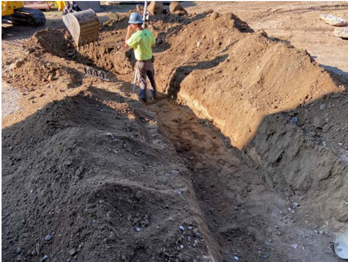
Trench excavation for fire alarm/telecom/IT conduits on south side (Part of PR#009)
