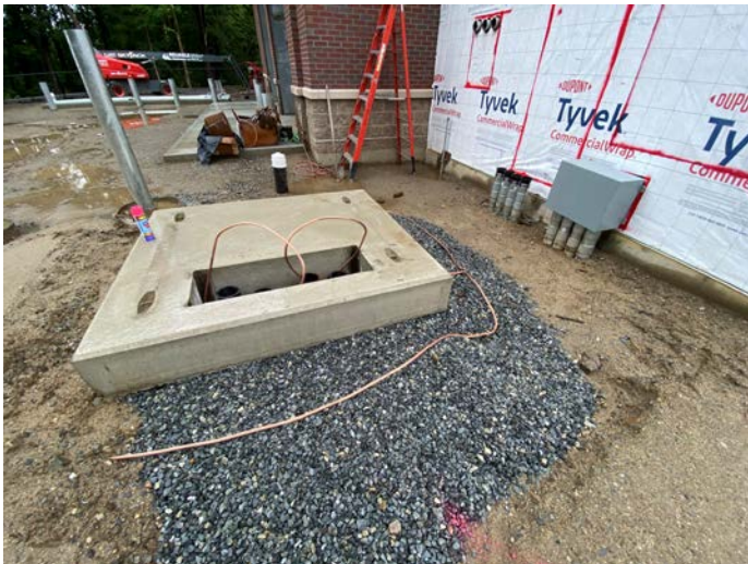
Transformer pad with grounding wires
