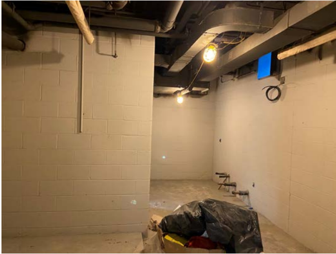
Block filler in dirty laundry room
