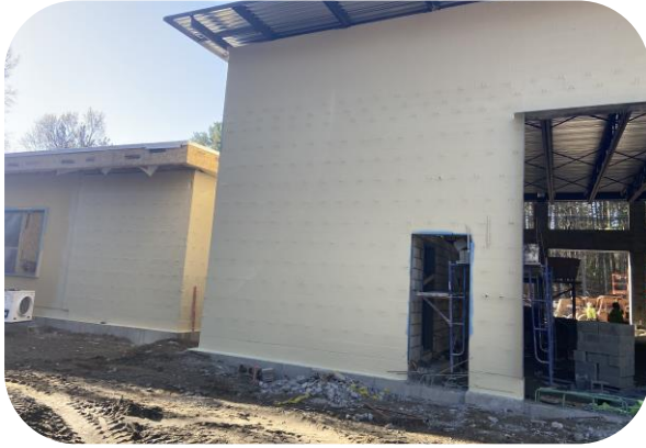
North side of apparatus bay with installed AVB
