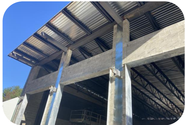
Sheet metal installed at steel columns on south face of apparatus bay for AVB preparation.
