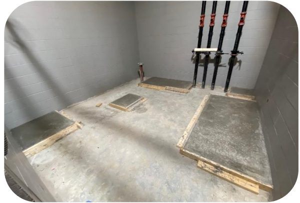
Mechanical pads installed in mechanical room
